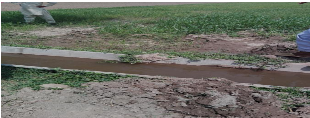
(Picture-1: Representing left side of watercourse was dismantled. This was done on the direction of local landlord to irrigate his fields illegally)
